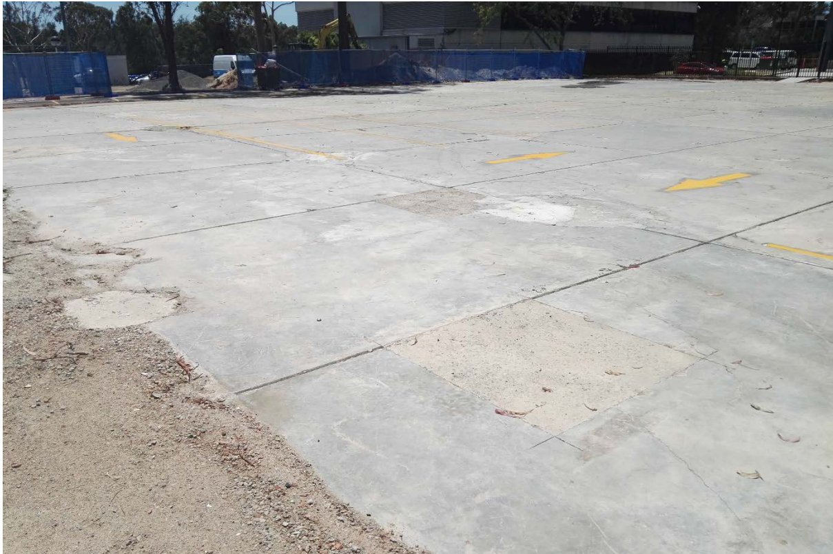
Photograph 4: Cracks and possible former service pits on the concrete slab
