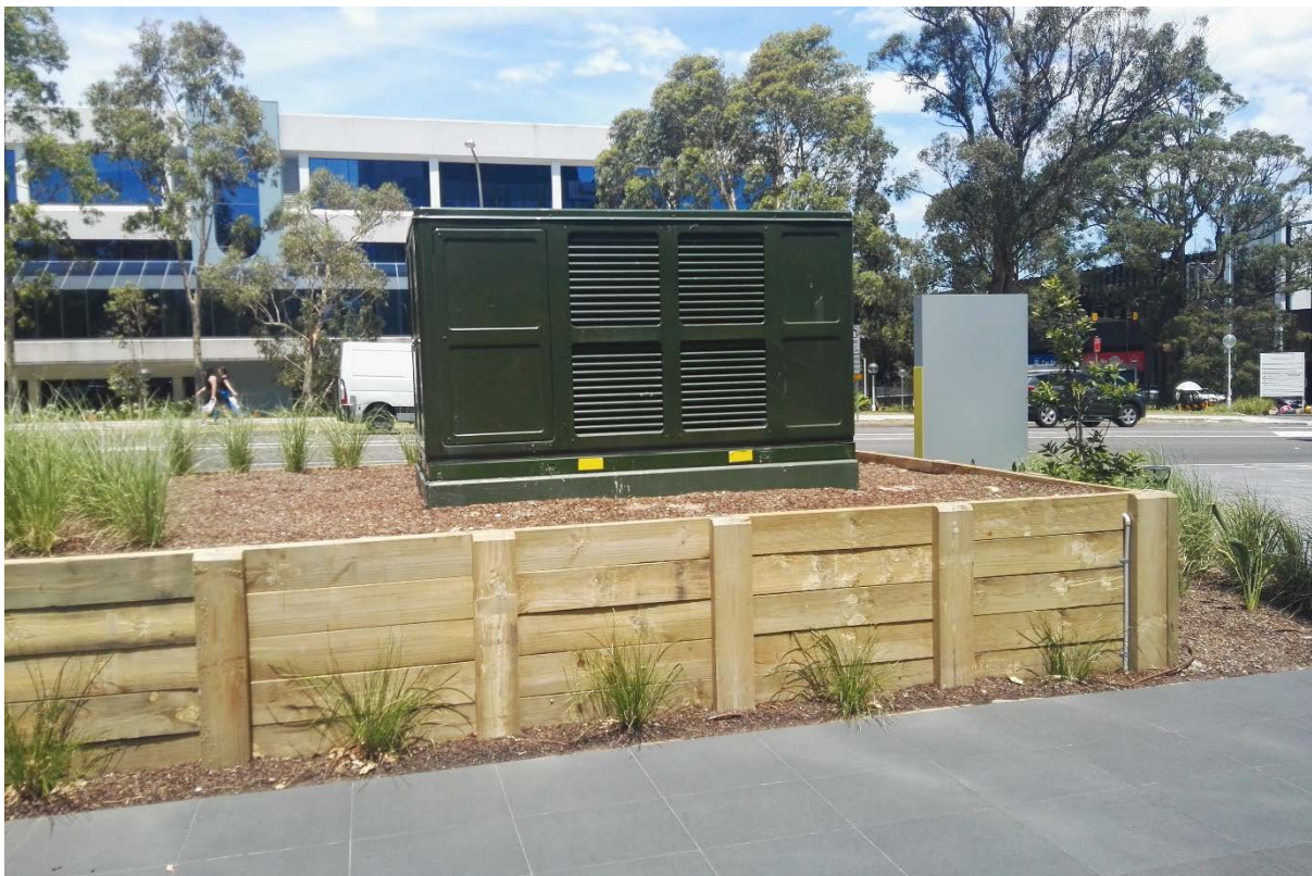
Photograph 9: On site substation
