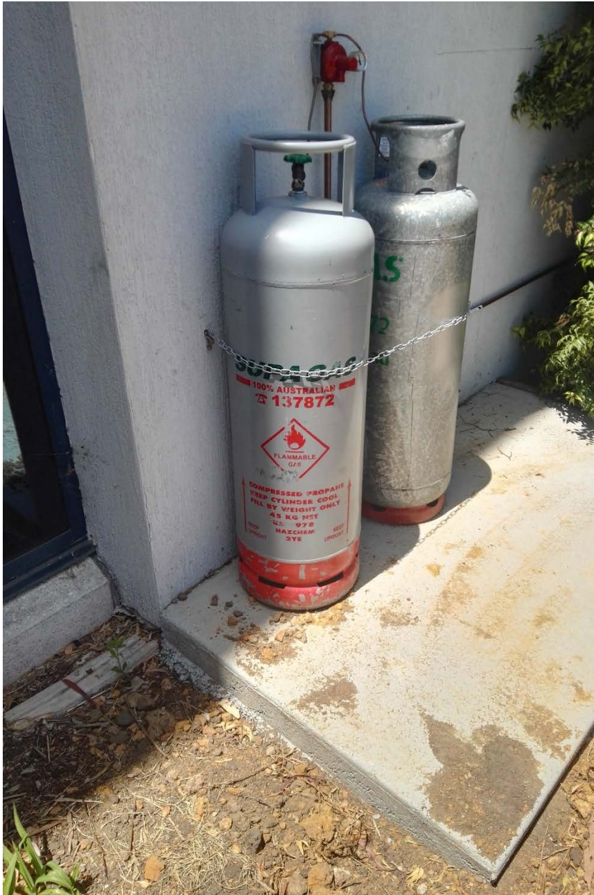
Photograph 12: Gas cylinders adjacent to the conference centre
